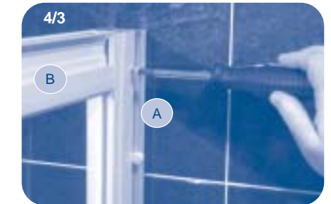
4/3 Screw provided screws into the new drilled holes at both bottom and top.
